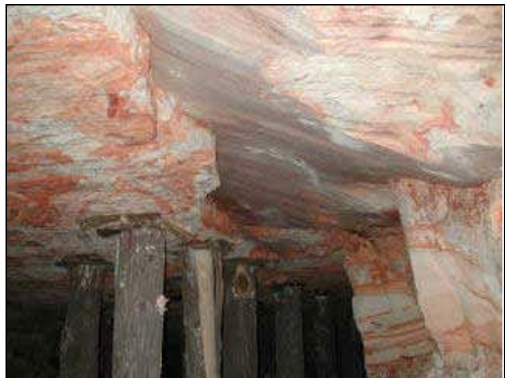
Fault plane (smooth surface) exposed in the sandstone roof of an opal mine, Coocoran opal fields, Lightning Ridge.
