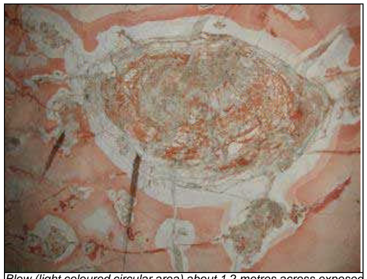
Blow (light coloured circular area) about 1.2 metres across exposed in the sandstone roof of a mine, Coocoran opal fields, Lightning Ridge.
